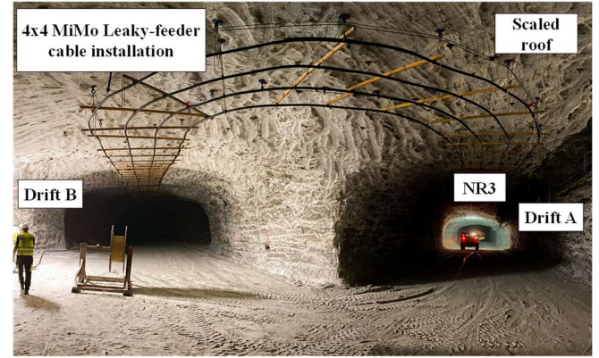
Fig. 7. Radiating cable setup at junction drift A, drift B in the underground mine site.
