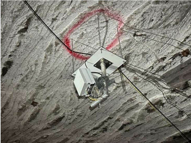
Fig. 6. Installation of 5G radio (NR2) in junction Drift A /Drift B, oriented to drift B (see Fig. 4).
